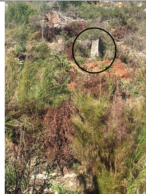
Figure 16: indicating the broken weir
