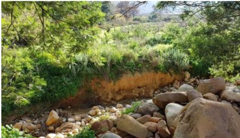
Figure 10: Photo showing site selected for the river crossing showing signs of degradation.
