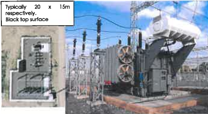
Figure 12: Transformer Pads and typical transformer
