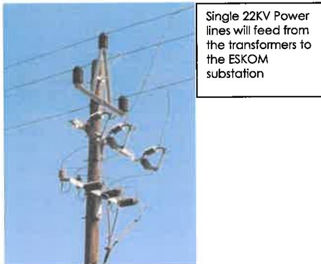
Figure 2: Typical 22kV Powerlines to connect to Taaibos Substation
