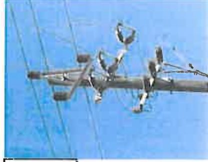
Figure 11: Typical 22KV single Power line
