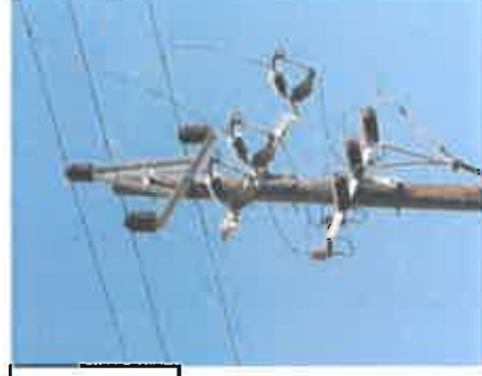
Figure 11: Typical 22KV single Power line
