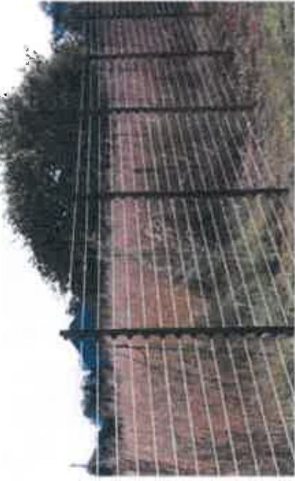
Figure 9: Typical electrical fence
