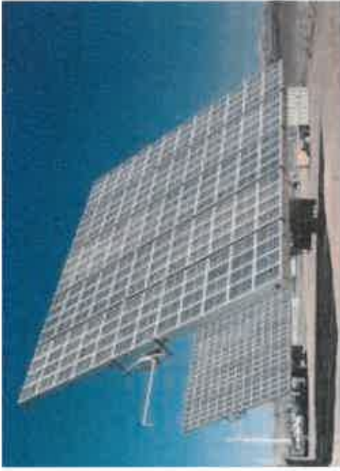
Figure 4: Typical CPV Unit
