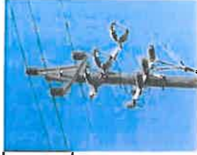
Figure 11: Typical 22KV single power line
