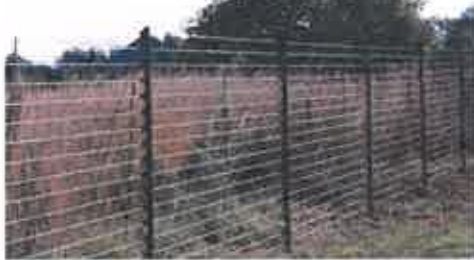
Figure 9: Typical electrical fence
