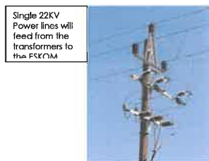
Figure 11: Typical 22KV single Powerline
