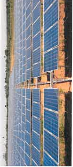
Figure 1: Single axis solar PV module tables raised 500mm above ground level
