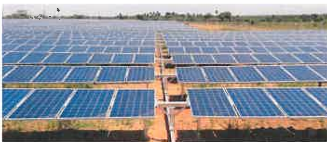
Figure 1: Single axis solar PV module tables raised 500mm above ground level
