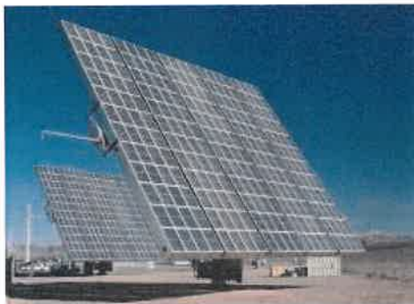
Figure 4: Typical CPV Unit
