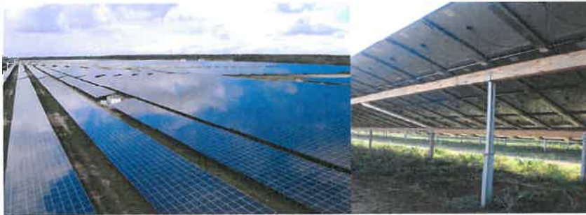
Figure 13: Example of PV arrays
