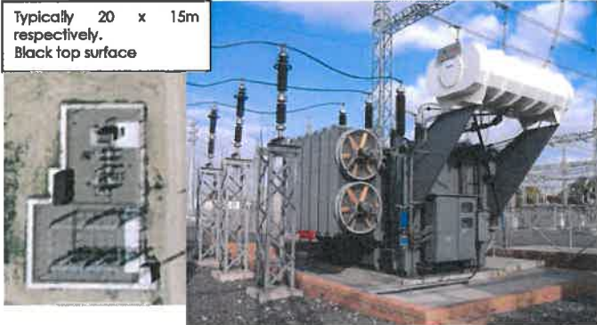
Figure 12: Transformer Pads and typical transformer
