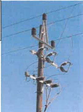
Figure 11: Typical 22KV single Powerline
