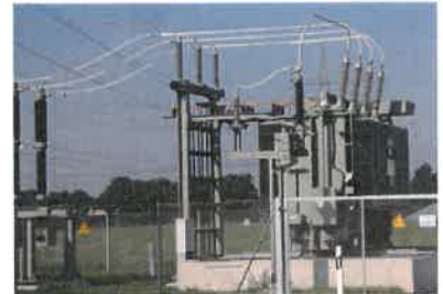
Figure 15: MV to HV Transformer
