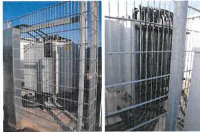
Figure 16: LV to MV Transformer station
