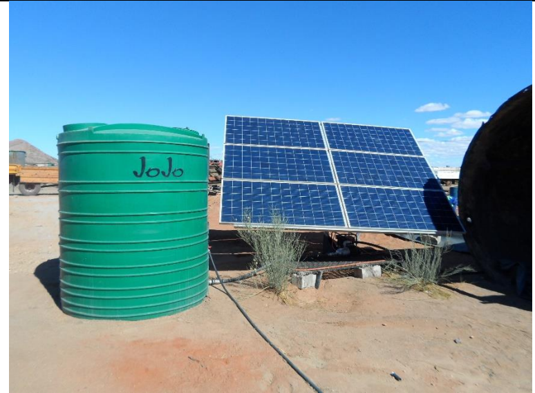
Figure 6: Pump station, powered by solar panels and JoJo tank used for the wet application
