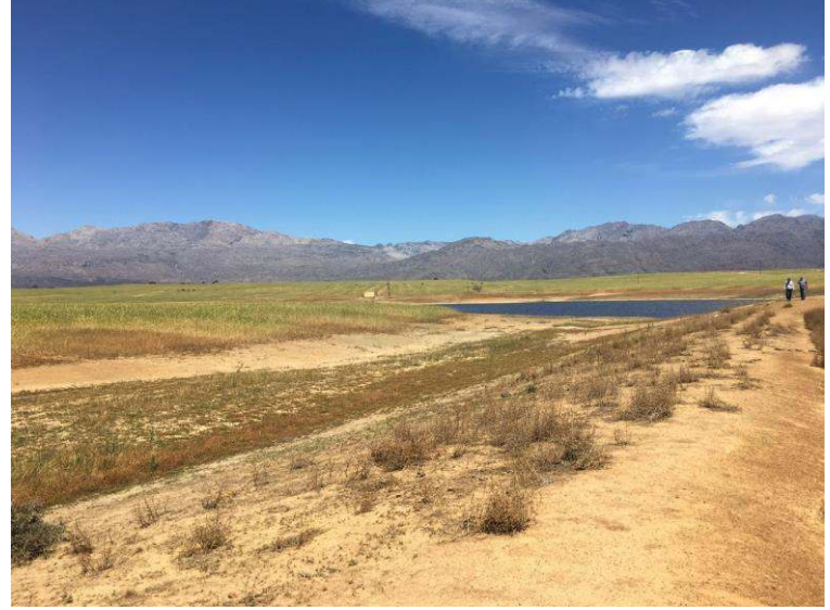
Figure 6: Photo taken from the far eastern part of the dam wall looking west towards to dam
