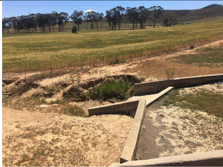
Figure 7: Spill way located on the north eastern part of the dam wall
