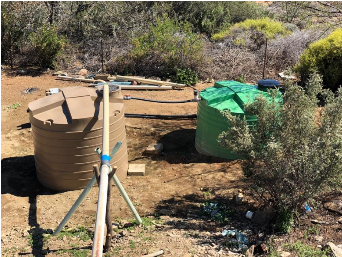
Figure 5: Chlorine contact tanks for treated effluent
