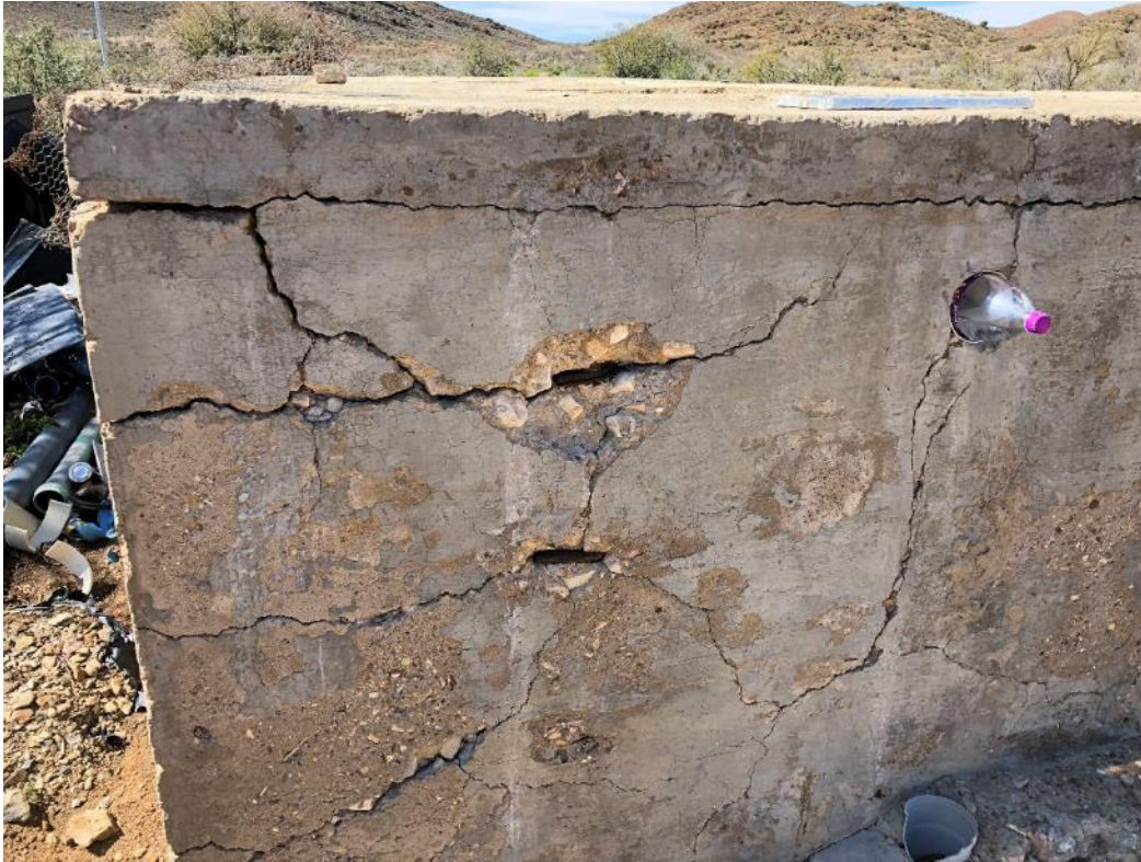
Figure 6: Existing Septic Tank structurally very unsound; not used
