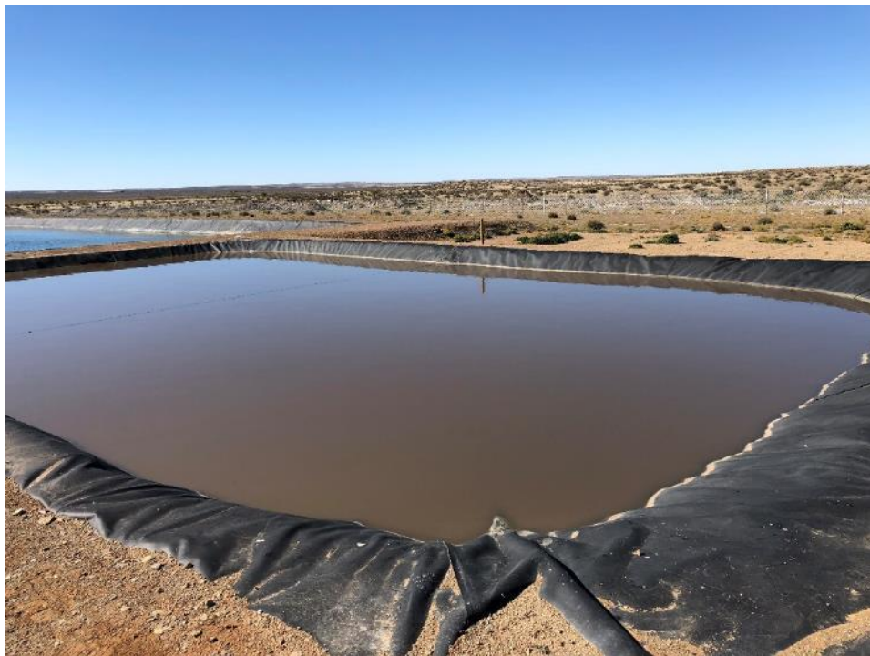
Typical Primary Anaerobic Pond with full HDPE Lining, Brandvlei Northern Cape
