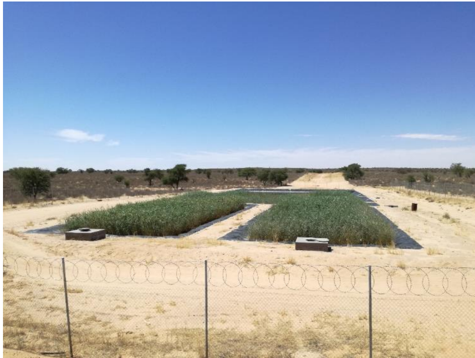
Typical Reedbed System: Nossob Rest Camp, Kgalagadi Transfronteir Park
