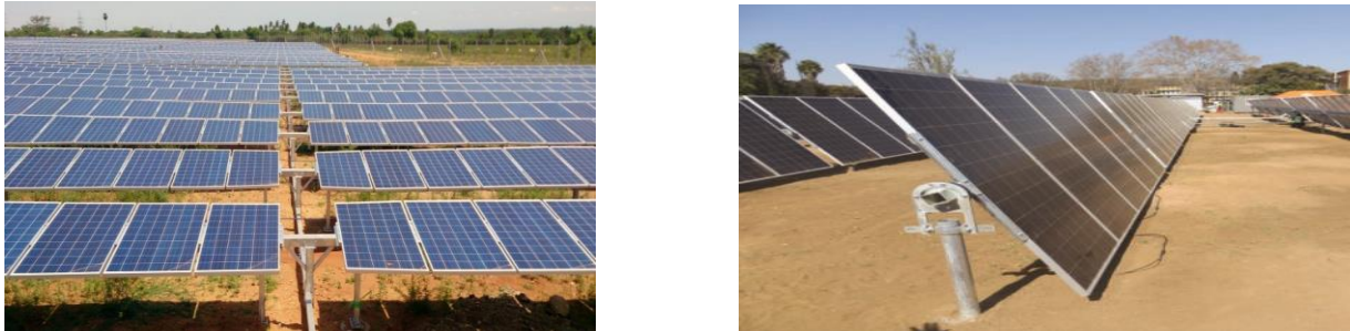
Figure 1: Single axis solar PV module tables raised 500mm above ground level (to a maximum tilt height of 3m).
