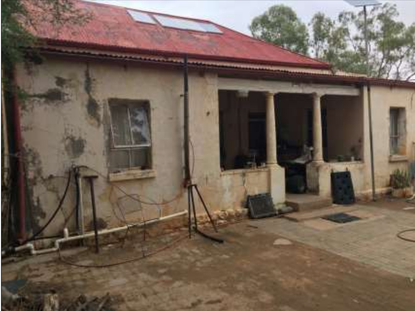
Figure 20. Farmhouse (main entrance). Note the alterations on the front stoep and steel windows. The enclosed stoep is a Victorian type feature.
