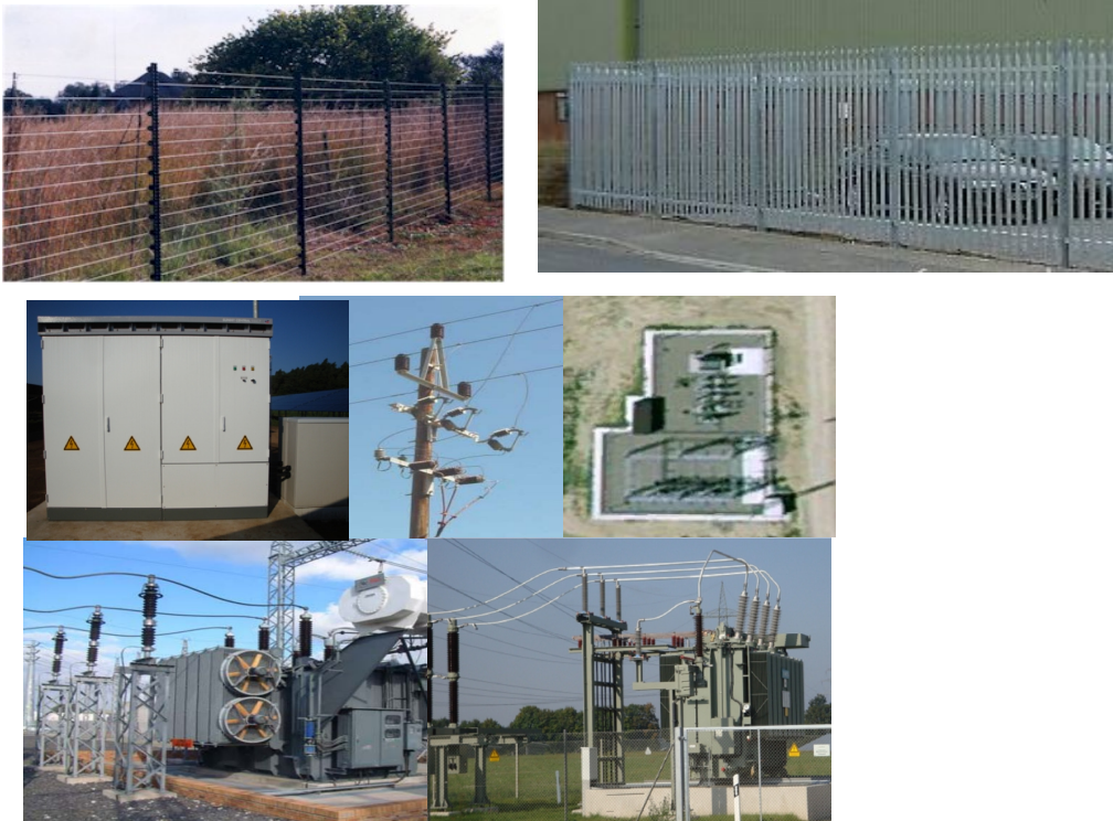
Figure 3: Typical support infrastructure i.e. power lines, substation & switches, fences
