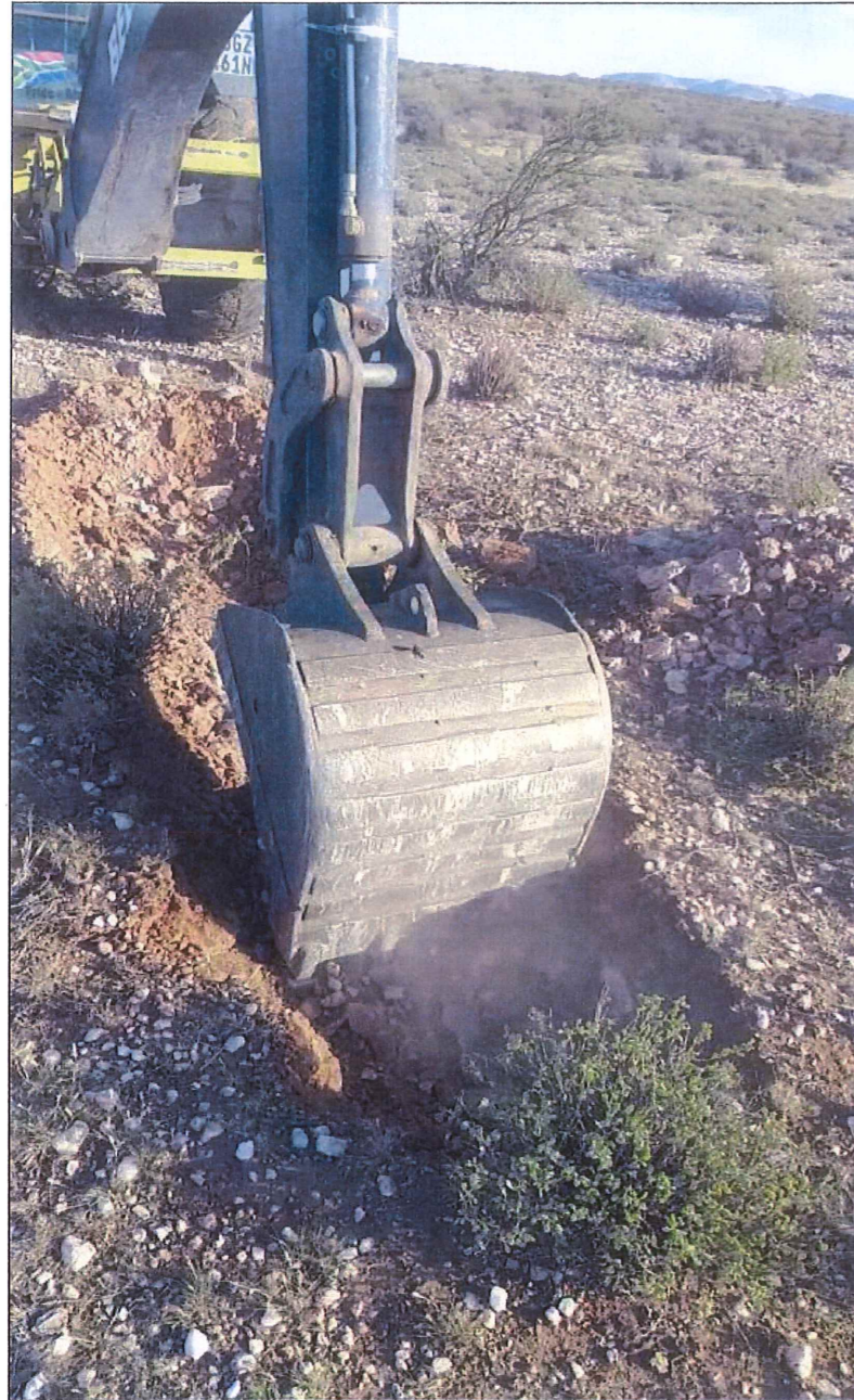
CONDITIONS OF REFUSAL OF EXCAVATION IN HARDPAN CALCRETE
