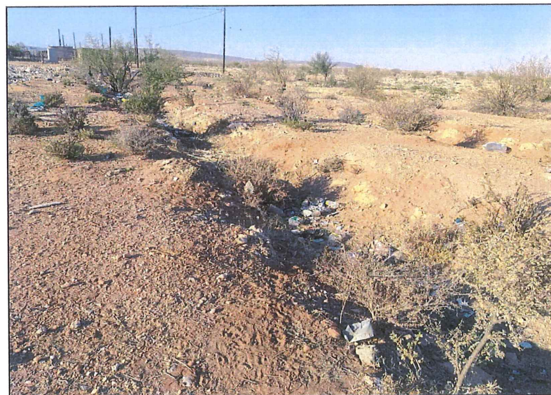
ABANDONED TRENCH EXCAVATIONS
