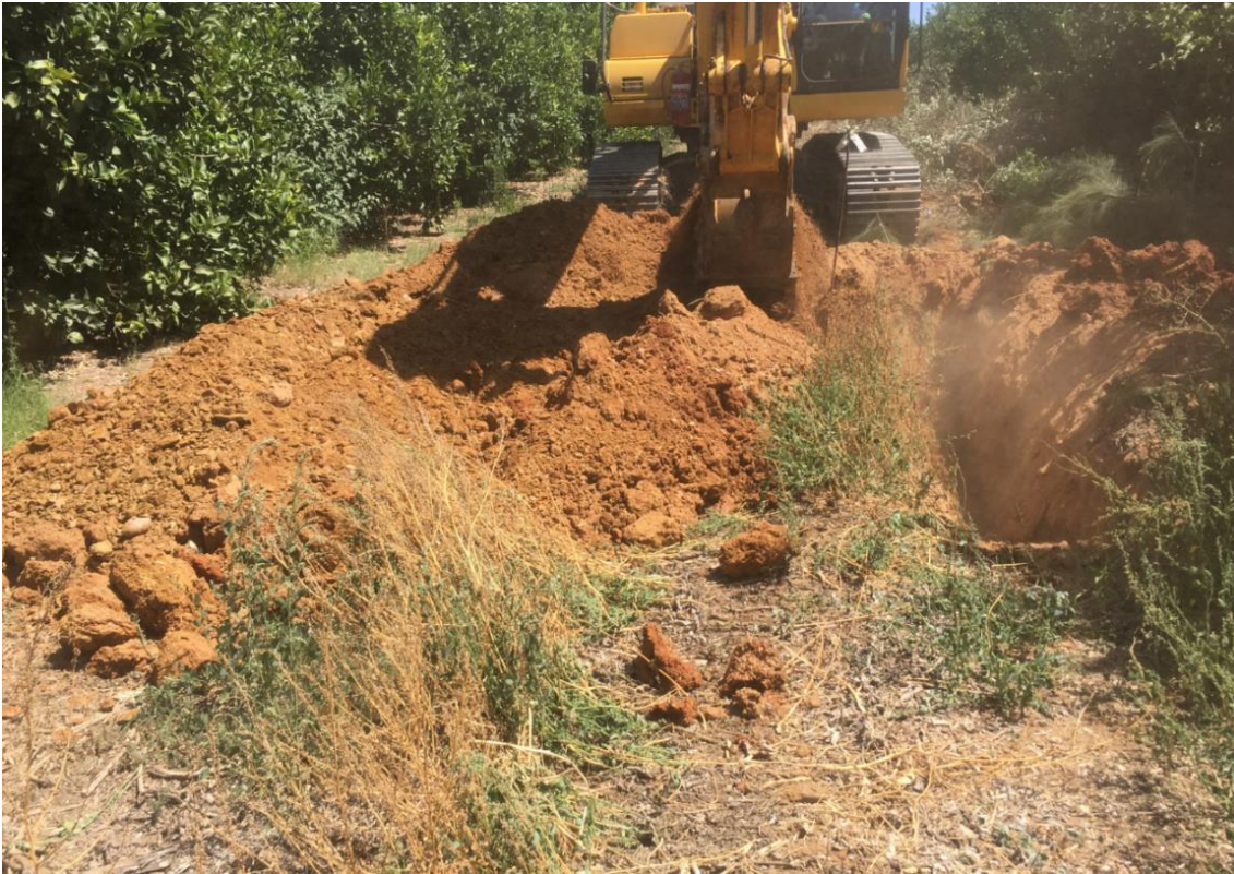
Figure 5-5: TP 1 located on the proposed embankment right flank below the embankment footprint
