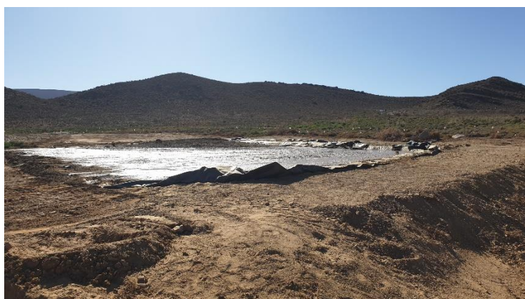
Sludge drying bed lined with plastic as per requirement
