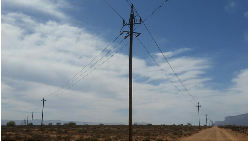
Photo 6: A photo showing a further view of the existing overhead lines in the vicinity of the proposed development (taken from position 2 in Figure 11)
