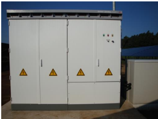
Figure 10: DC to AC inverter Interface
