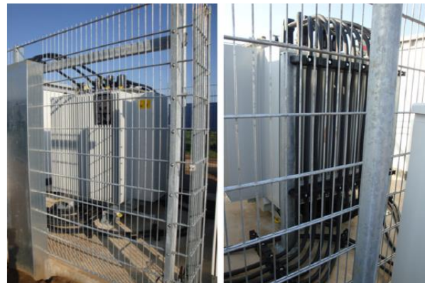
Figure 12: LV to MV Transformer station
