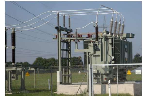
Figure 11: MV to HV Transformer
