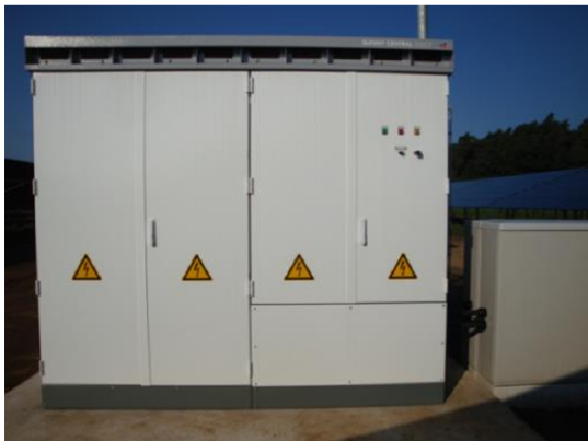
Figure 10: DC to AC inverter Interface
