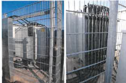
Figure 16: LV to MV Transformer station
