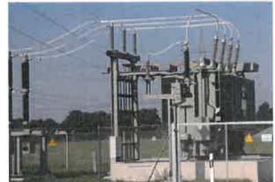
Figure 15: MV to HV Transformer
