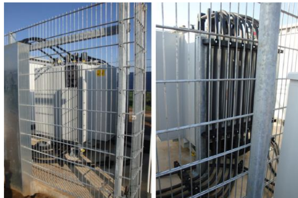
Figure 12: LV to MV Transformer station
