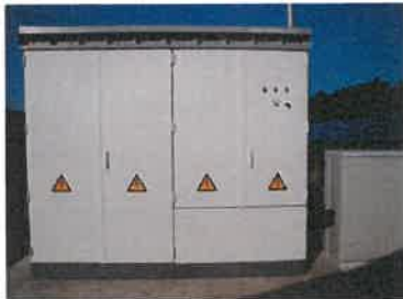
Figure 14: DC to AC Inverter Interface
