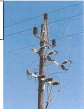
Figure 11: Typical 22KV single Powerline
