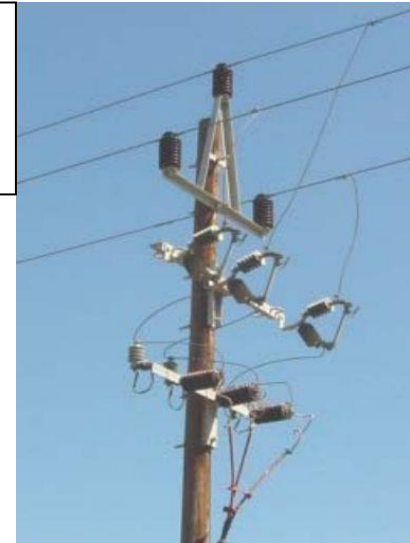
Figure 7: Typical 22KV single Powerline
