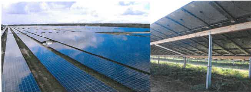
Figure 13: Example of PV arrays
