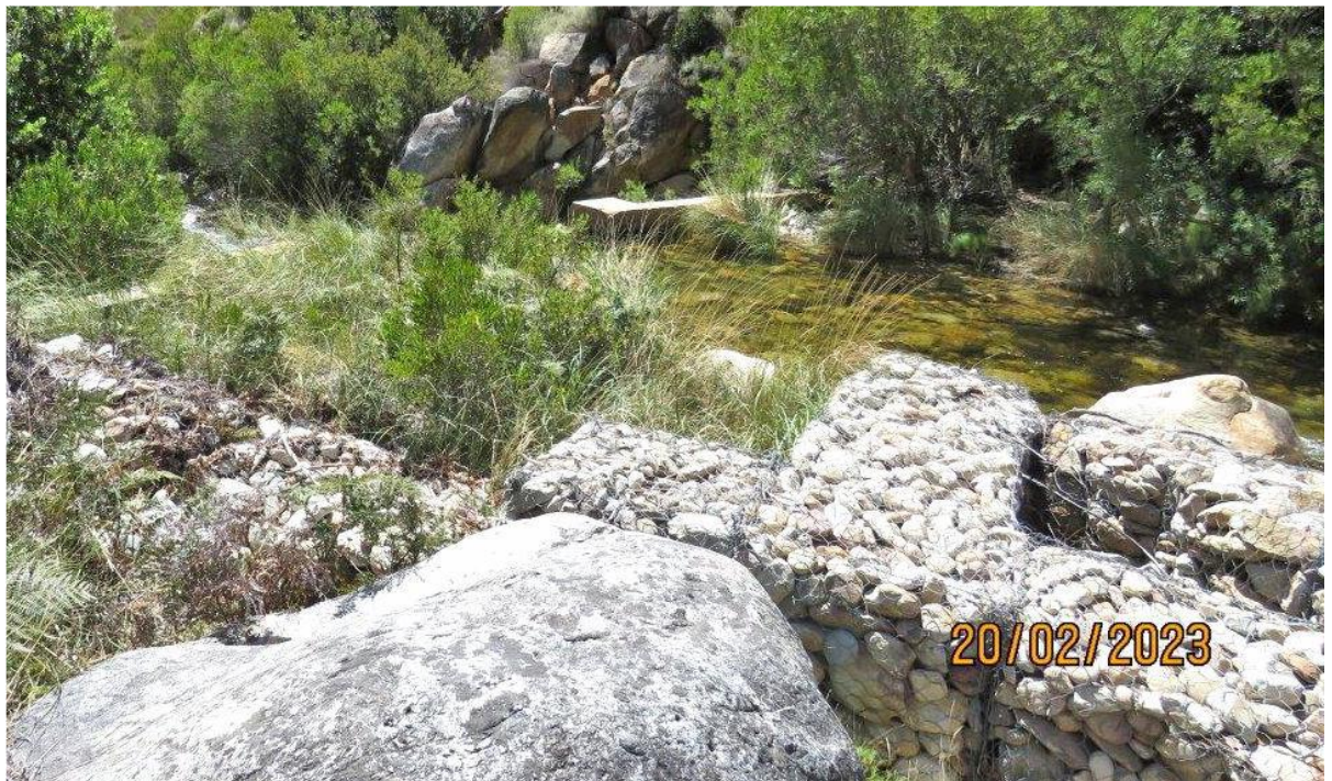
Photo 2: View of gabions at the weir where abstraction in the Tierhokskloof Stream takes place
