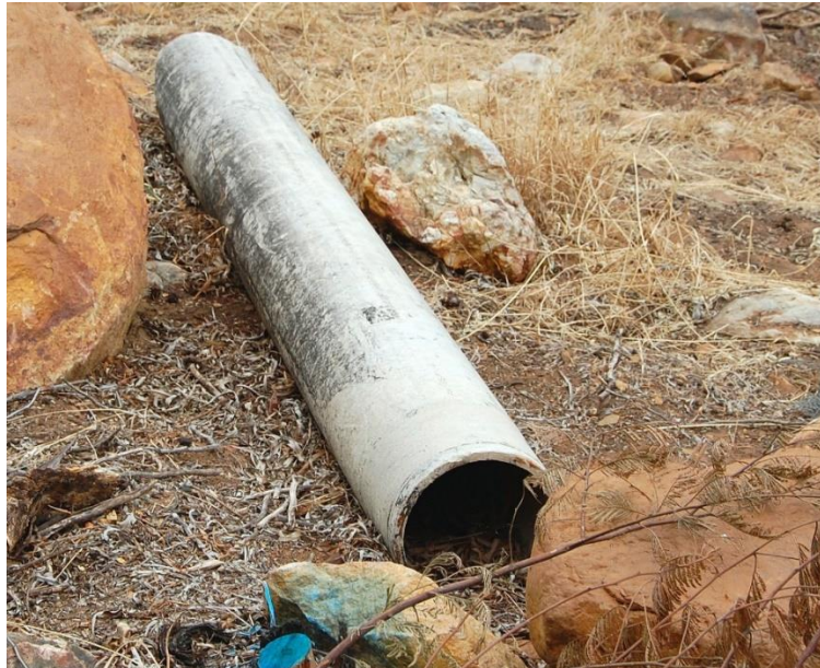
Figure 9 Broken section of pipe
