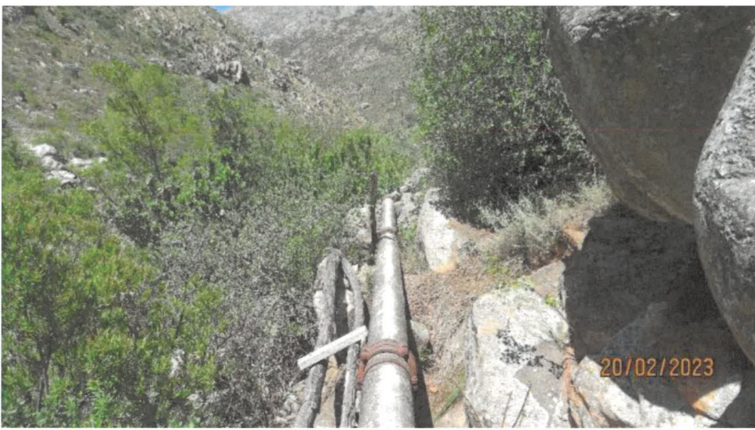
Photo 1: West to east view of the proposed site showing the existing bulk water supply pipeline
