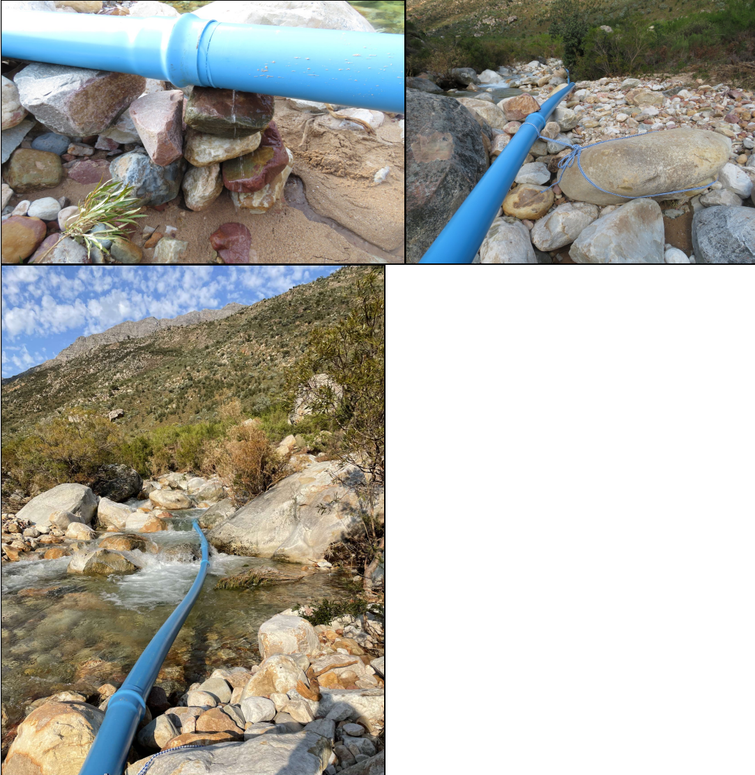
Plates 1a, 1b and 1c: Photographs near weir of blue plastic pipe which is precariously placed and needs to be replaced with a pipeline that blends into the environment. It is not clear when this blue pipeline was installed.
