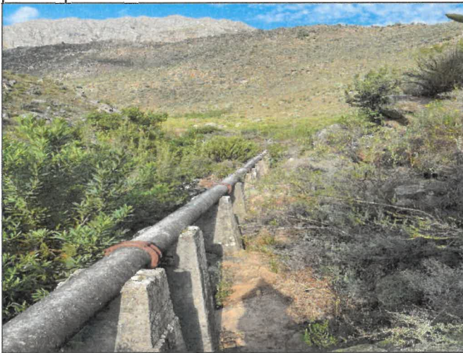
Plate 3: The existing support structures are quite substantial and should be reused if possible to minimise disturbance and reduce rubble that has to be removed from site. No additional structure should be built on the river side of the existing structures.
