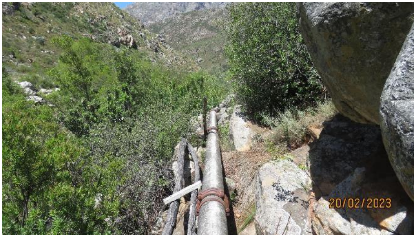
Photo 5: Another of the narrow rocky area, slightly further north (downstream from Picture 3) where the pipeline will have to be placed (most likely to the left of the existing pipeline).
