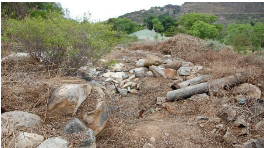
Photo 15: The WTW is located on a small rocky outcrop near Witbrug. The photo shows the disturbed footprint area where pipelines had to be replaced (as it goes up this rocky outcrop).
