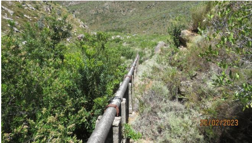
Photo 4: One of the narrow rocky areas (looking from the north to south into the Tierhokskloof) in the Tierhokskloof, downstream of the inlet structure. Note the larger trees e.g., Heeria and Brabejum , towards the river (to the left of picture). Some of these trees might have to be trimmed.
