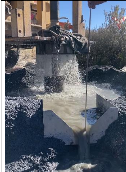
Airlift yield of 1800 L/h (0.5 L/s) at borehole MAR 5.
