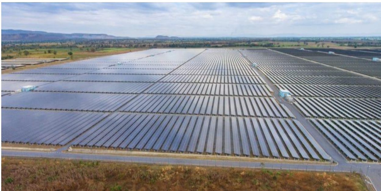
Figure 5: Perimeter Fencing around a Solar PV Facility
