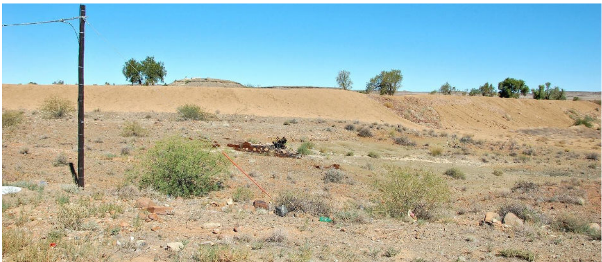
Photo 3: View of the wall of the dam located approximately 100m south of proposed site
