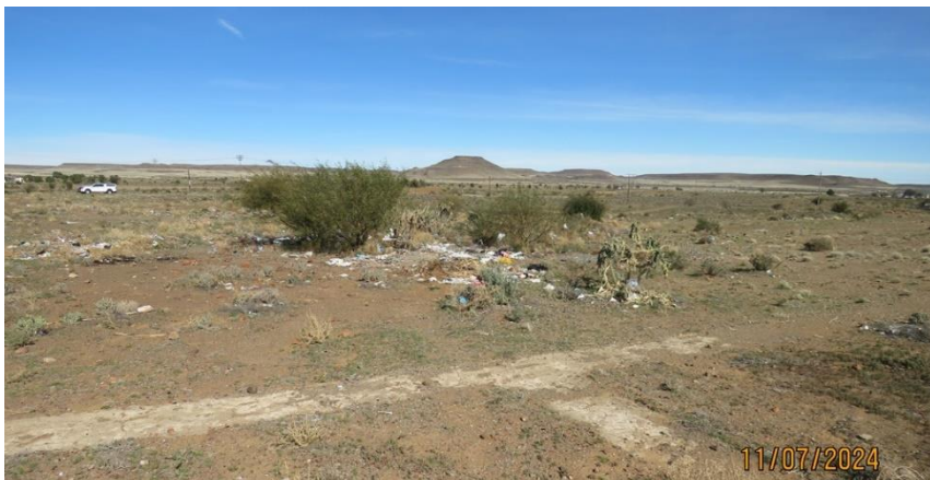
Photo 6: Building foundations showing in the foreground. Prosopis trees and the alien Harrisia martini (toukaktus) and illegal dumping can be observed in the middle of picture.
