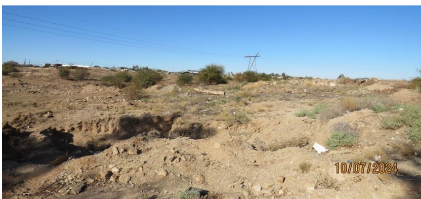
Photo 6: Looking from west to east over the site. Excavations can be seen in the foreground and the Eskom overhead cables in the background.
