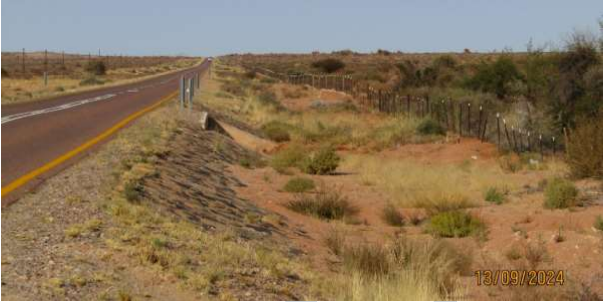
Photo 2: An example of a drainage line crossing with a culvert along the R27. Vegetation comprising woody species such as Vachellia karoo and the alien Prosopis sp. occurring just outside the road reserve
