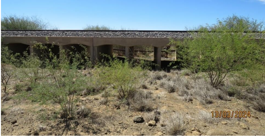
Photo 44: Culvert underneath the Sishen-Saldana railway line, through which the pipeline will cross.
