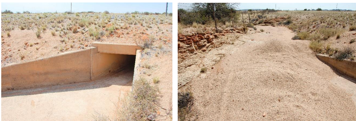
Figure 35 Point No.15 crossing
