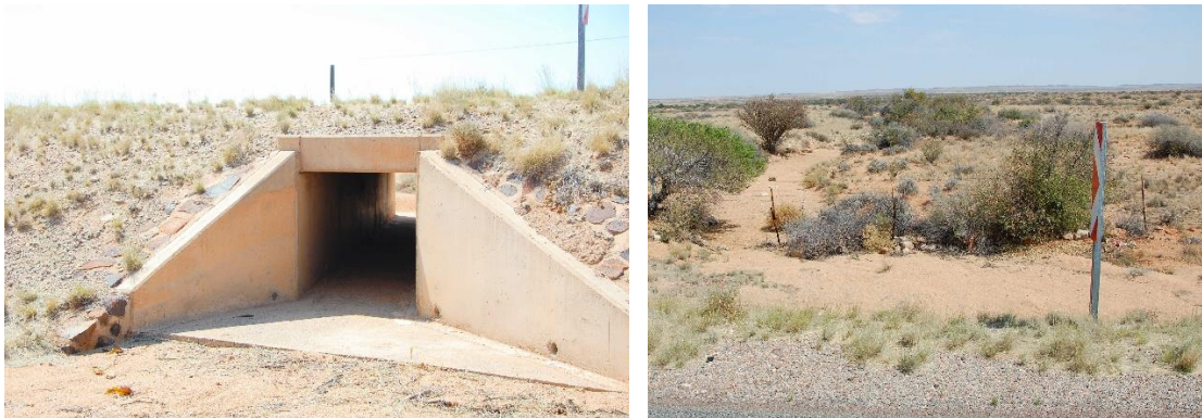
Figure 34 Point No.14 crossing
