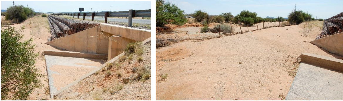
Figure 36 Point No.17 crossing
