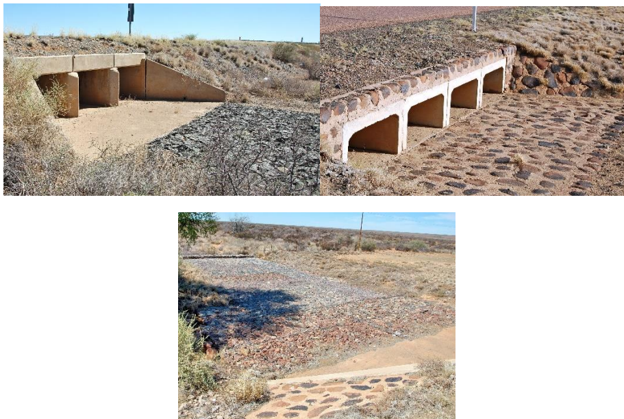
Figure 56 Stormwater calming infrastructure.
