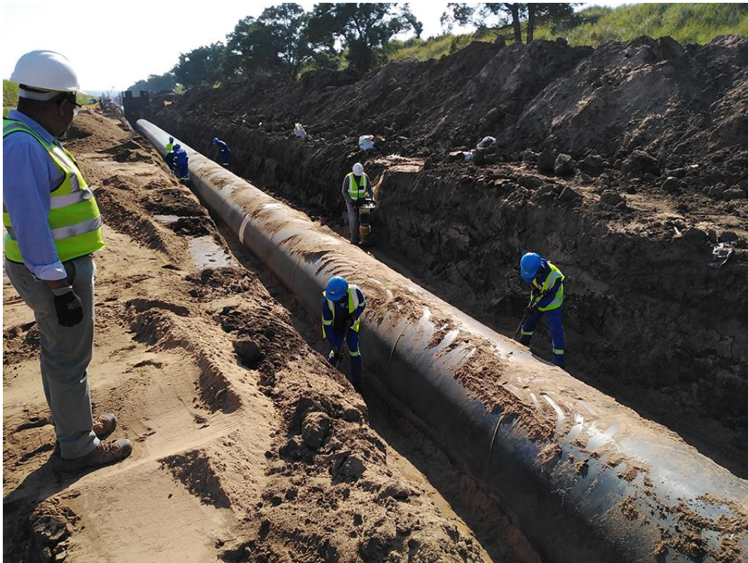
Figure 5: Raw Water Pipeline in Richards Bay
