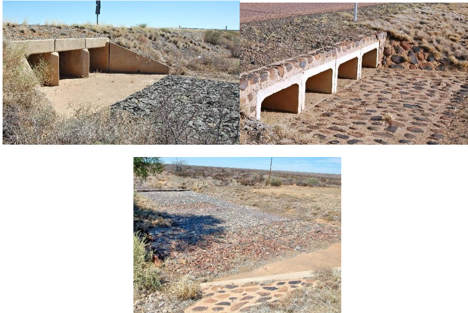
Figure 14 Stormwater calming infrastructure.
