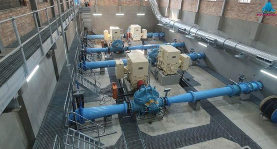
Figure 4: Riverton Pumpstation, Kimberley, Northern Cape
