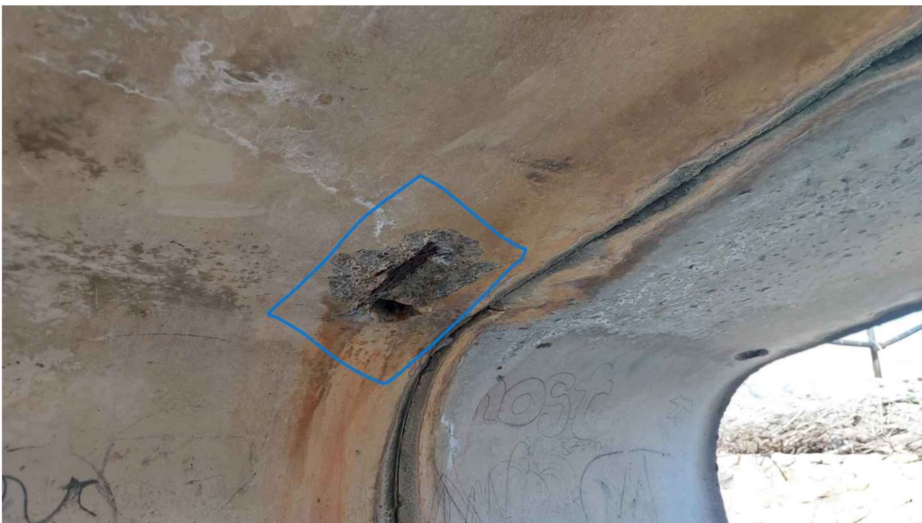
PHOTO 2: EXPOSED REINFORCEMENT TO BE REPAIRED
