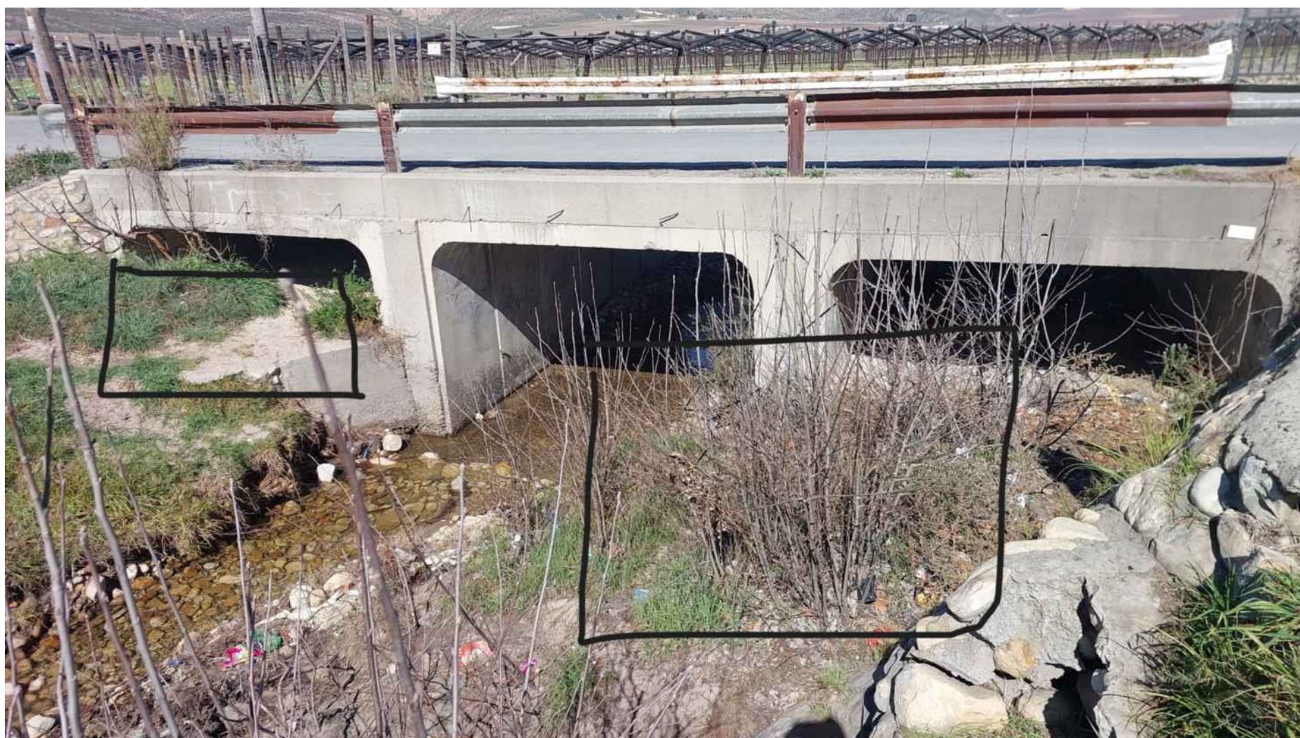
PHOTO 3: DEBRIS ACCUMULATION TO BE REMOVED AND CLEAR WATERWAY
