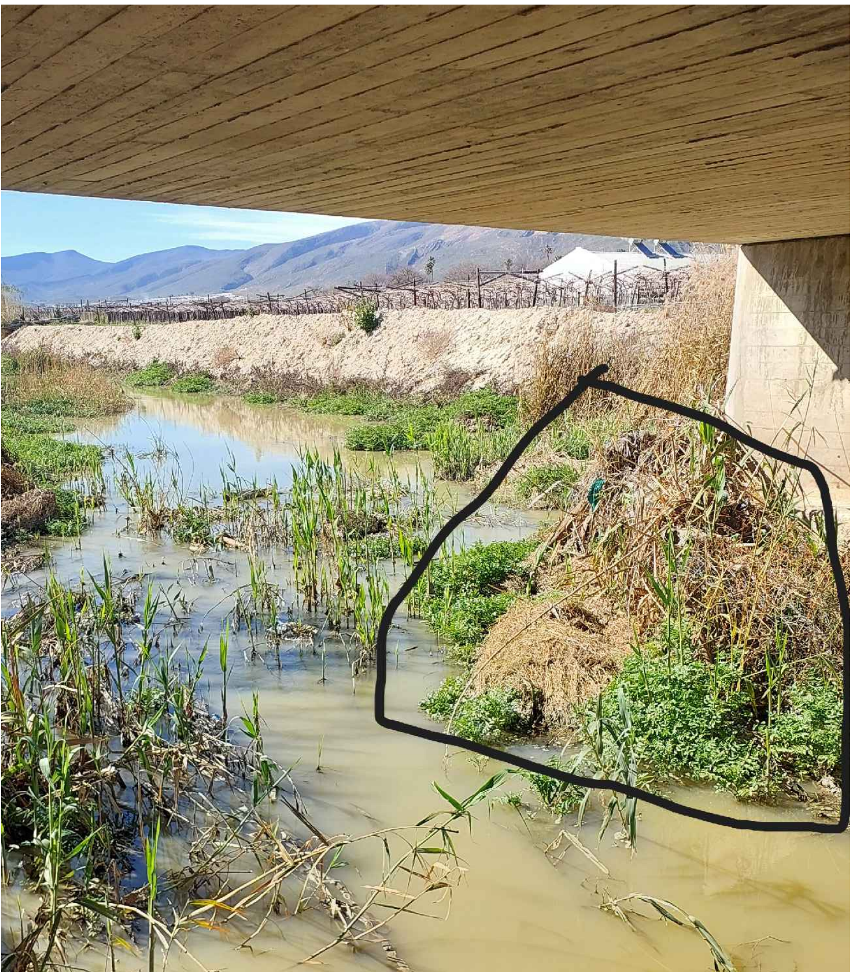
PHOTO 1: DEBRIS ACCUMULATION TO BE REMOVED AND CLEAR WATERWAY
