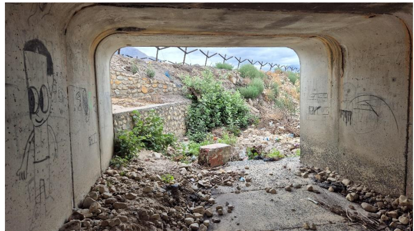
Photo 4: Photograph of accumulated material to be cleared from chamber of culvert
