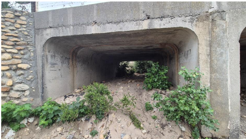
Photo 3: Photograph of accumulated material to be cleared from chamber of culvert
