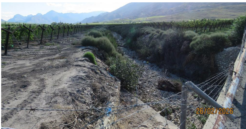
Photo 6: The severely degraded outlet wing of Culvert 10432. Note the general degraded status and woody invasive species.
