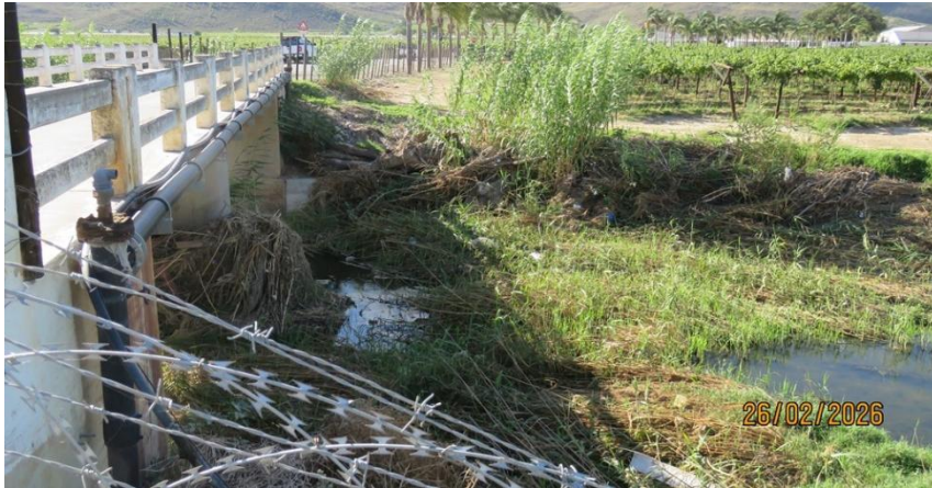
Photo 3: Hex River. The inlet of the small bridge over the Hex River. Note the severely degraded state of the river.
