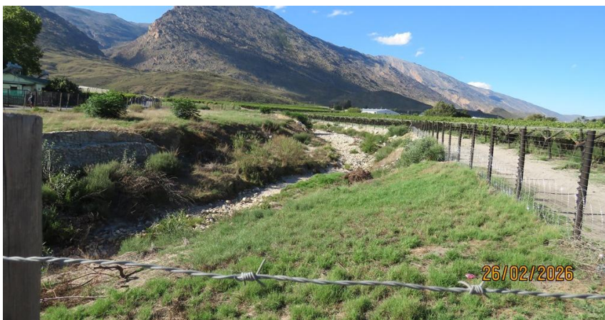
Photo 5: The severely degraded inlet wing of Culvert 10432. Note the general degraded status.
