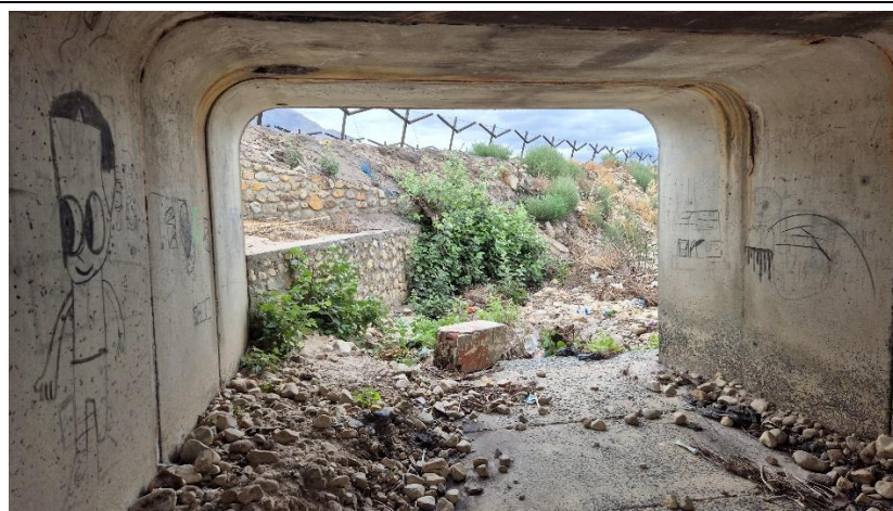
Photo 4: Photograph of accumulated material to be cleared from chamber of culvert
